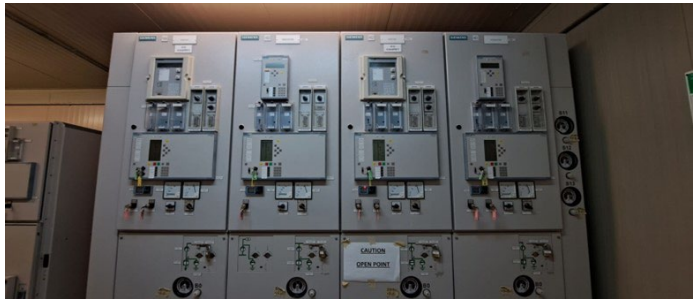
33KV MV SWITCHGEAR PANEL AT AL MARKAZ INDUSTRIAL PARK, DHFRAH
