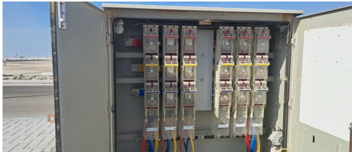
FEEDER PILLAR AT AL MARKAZ INDUSTRIAL PARK, AL DHAFRAH
