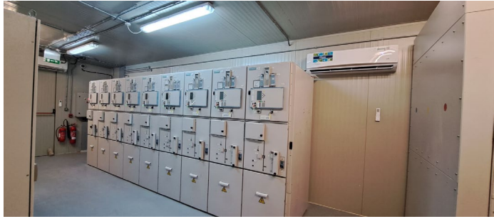
11KV MV SWITCHGEAR PANEL AT AL MARKAZ INDUSTRIAL PARK, DHFRAH
