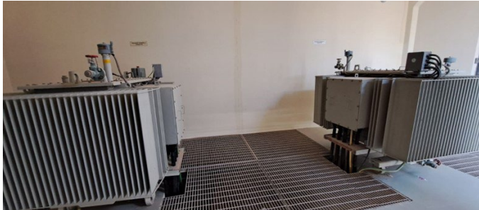
TRANSFORMER AT 110.415KV DISTRIBUTION SUBSTATION, AL MARKAZ INDUSTRIAL PARK, DHFRAH
