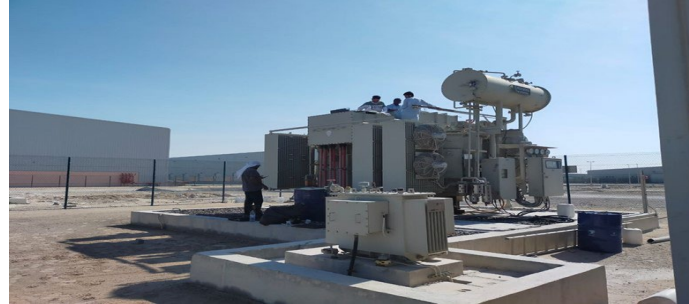
33/11KV KV TRANSFORMER OIL LEAKAGE RECTIFICATION & OIL FILLING AT AL MARKAZ INDUSTRIAL PARK, DHFRAH
