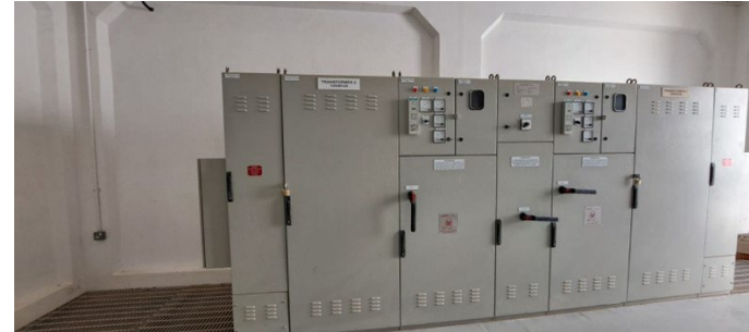
LV PANEL AT DISTRIBUTION SUBSTATION, AL MARKAZ INDUSTRIAL PARK, DHFRAH
