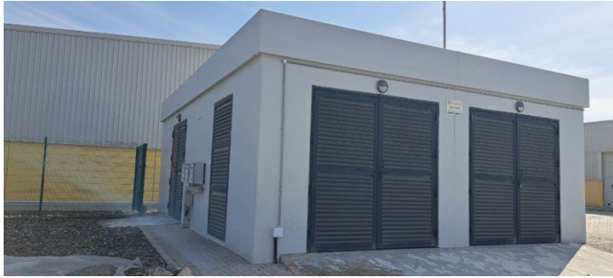
110.415KV DISTRIBUTION SUBSTATION, AL MARKAZ INDUSTRIAL PARK, DHFRAH
