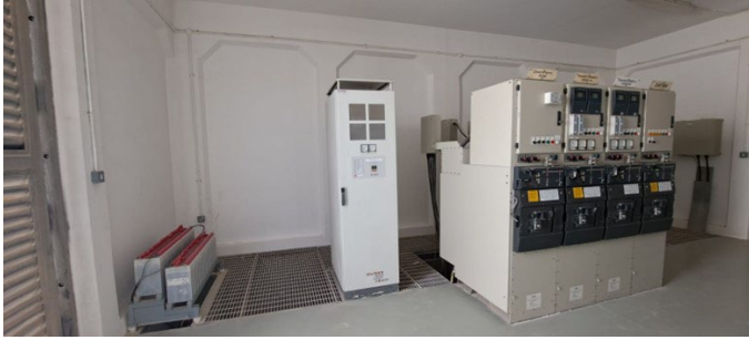
11KV MV SWITCHGEAR PANEL & DC CHARGER PANEL AT DISTRIBUTION SUBSTATION, AL MARKAZ INDUSTRIAL PARK, DHFRAH
