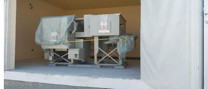
GRM AT SUBSTATION, PROJECT: COSMOPLAST FACILITIES AT KIZAD
