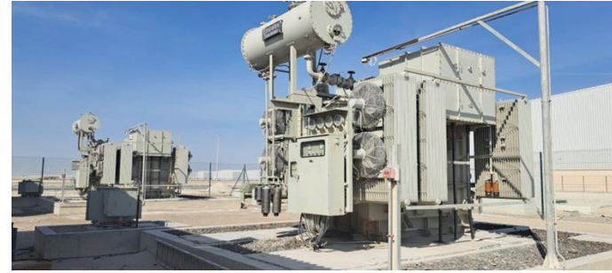
33/11KV KV TRANSFORMER AT AL MARKAZ INDUSTRIAL PARK, DHFRAH
