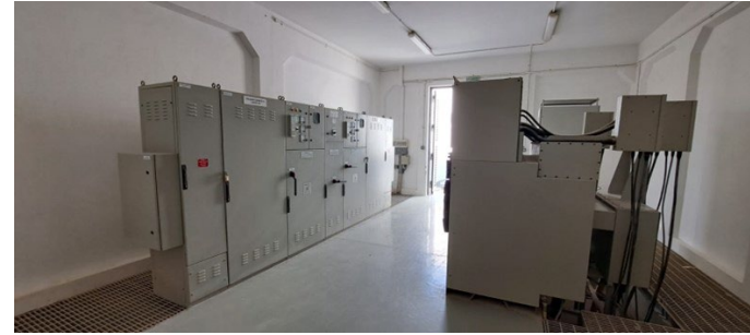
MV SWITCHGEAR ROOM AT DISTRIBUTION SUBSTATION, AL MARKAZ INDUSTRIAL PARK, DHFRAH
